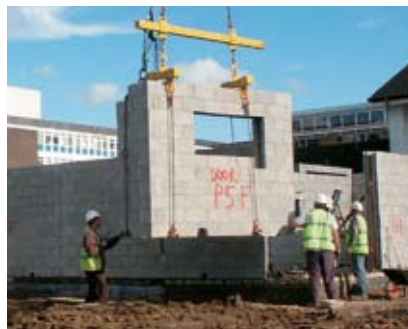
Construction of Hanson demonstration house for OFFSITE2007 – Hanson's OFFSITE2007 house will address climate change issues
