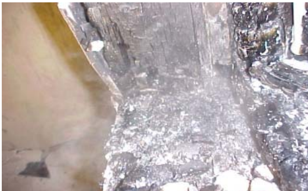
Photograph C12. Showing post test damage.
