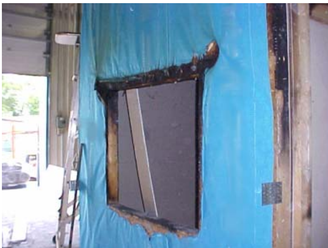
Photograph C13. Showing post test damage.
