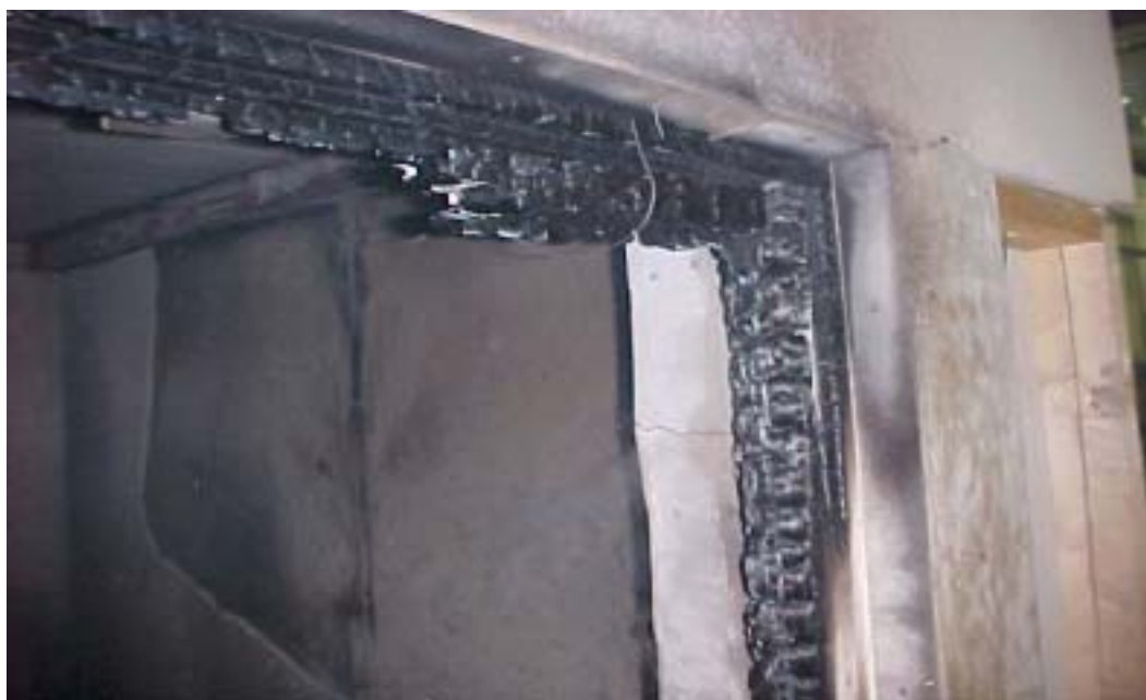
Photograph C10. Showing post test damage.
