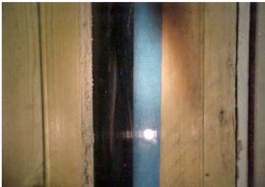
Photograph C3. Showing distortion of the window frame.
