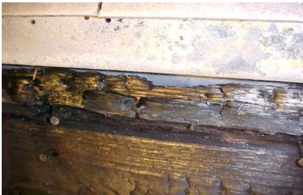
Photograph C2. Showing post test damage.
