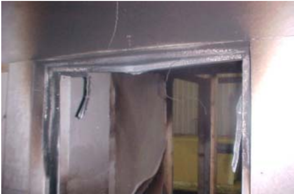
Photograph C6. Showing post test damage.
