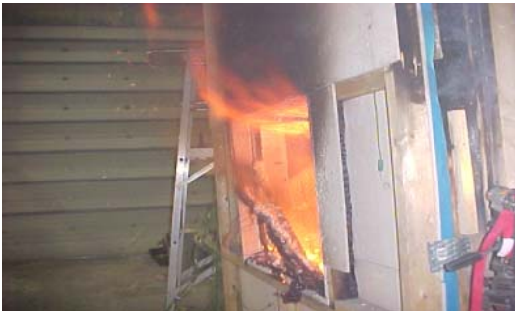
Photograph C1. Showing the break through of flames out of the enclosure
