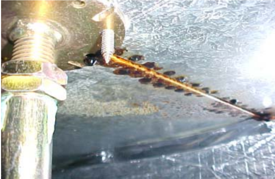
Photograph A11. Shows damage to an exposed floor panel.
