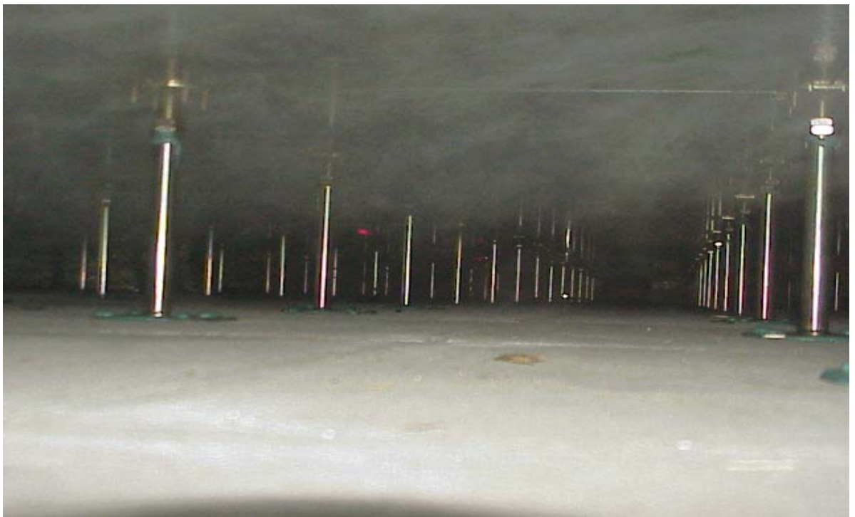
Photograph A8. Smoke on the unexposed side of the barrier.
