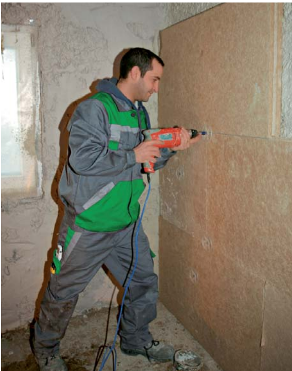
Figure 5: Fixing wood fibre insulation boards to existing internal walls (Courtesy of Natural Building Technologies)
