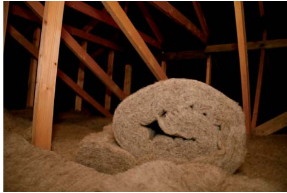
Figure 6: Natural fibre insulation is non-toxic and there is generally no requirement for protective clothing or respirators during installation (Courtesy of Black Mountain Insulation)
