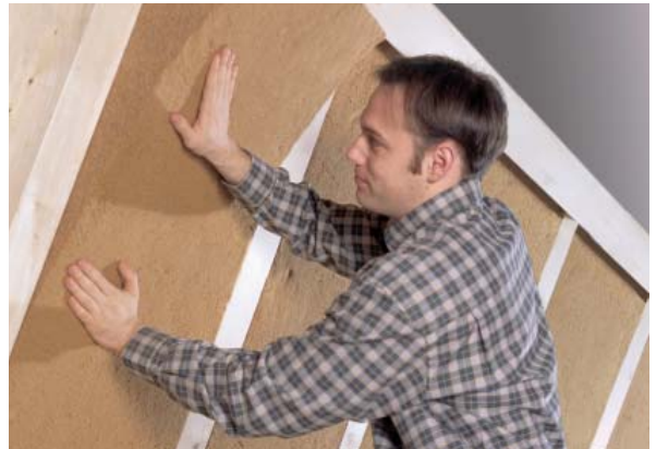
Figure 2: Fibre boards being fitted between timber battens (Courtesy of Natural Building Technologies)
