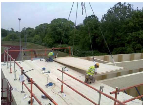
Figure 5: Installation of CLT floor panels – the construction environment is relatively free from noise and dust (Courtesy of KLH)
