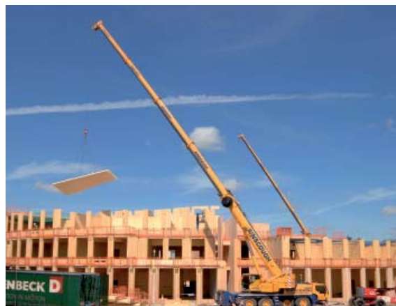
Figure 7: CLT panels being lifted into position – construction should be fast compared with most traditional methods, although additional resources may be needed in the planning and design stages
