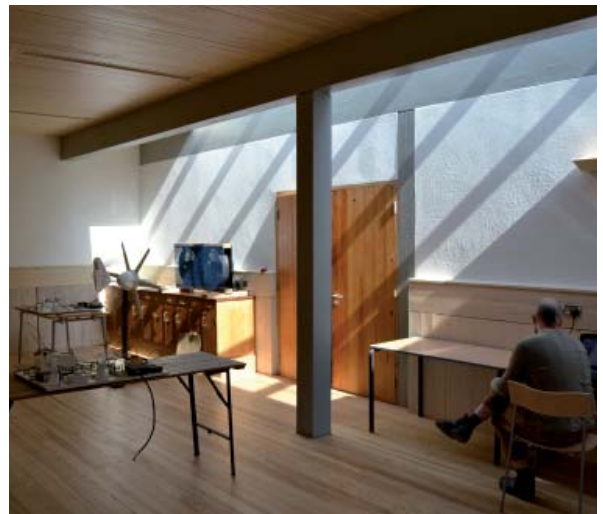
Figure 1: Internal rendered partition walls using unfired clay block at Wales Institute for Sustainable Education (WISE), Centre for Alternative Technology (CAT), Machynlleth
