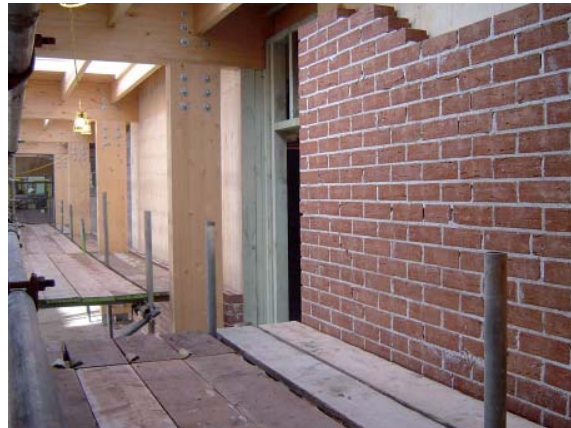
Figure 7: Unfired clay brick walling at Neal's Yard, Dorset (Courtesy of Feilden Clegg Bradley Studios)
