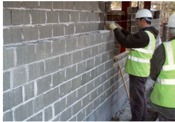
Figure 2: Unfired clay bricks can easily be laid by bricklayers with little or no further training (Courtesy of Ecoterre)
