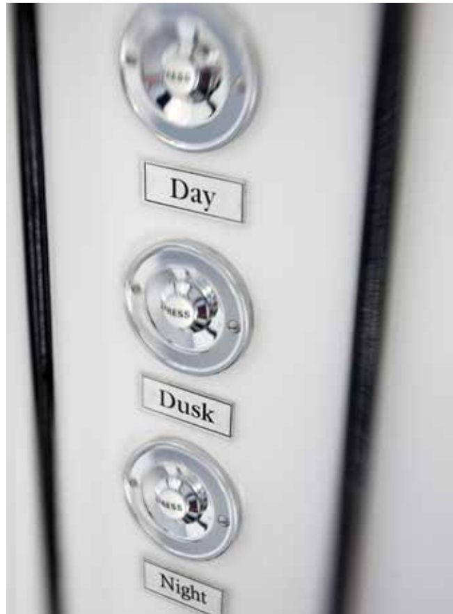
Figure 40: Flexible controls allowing shoppers to change lighting settings in the fitting rooms, between simulated 'day', 'dusk' and 'night' (© Boux Avenue)
