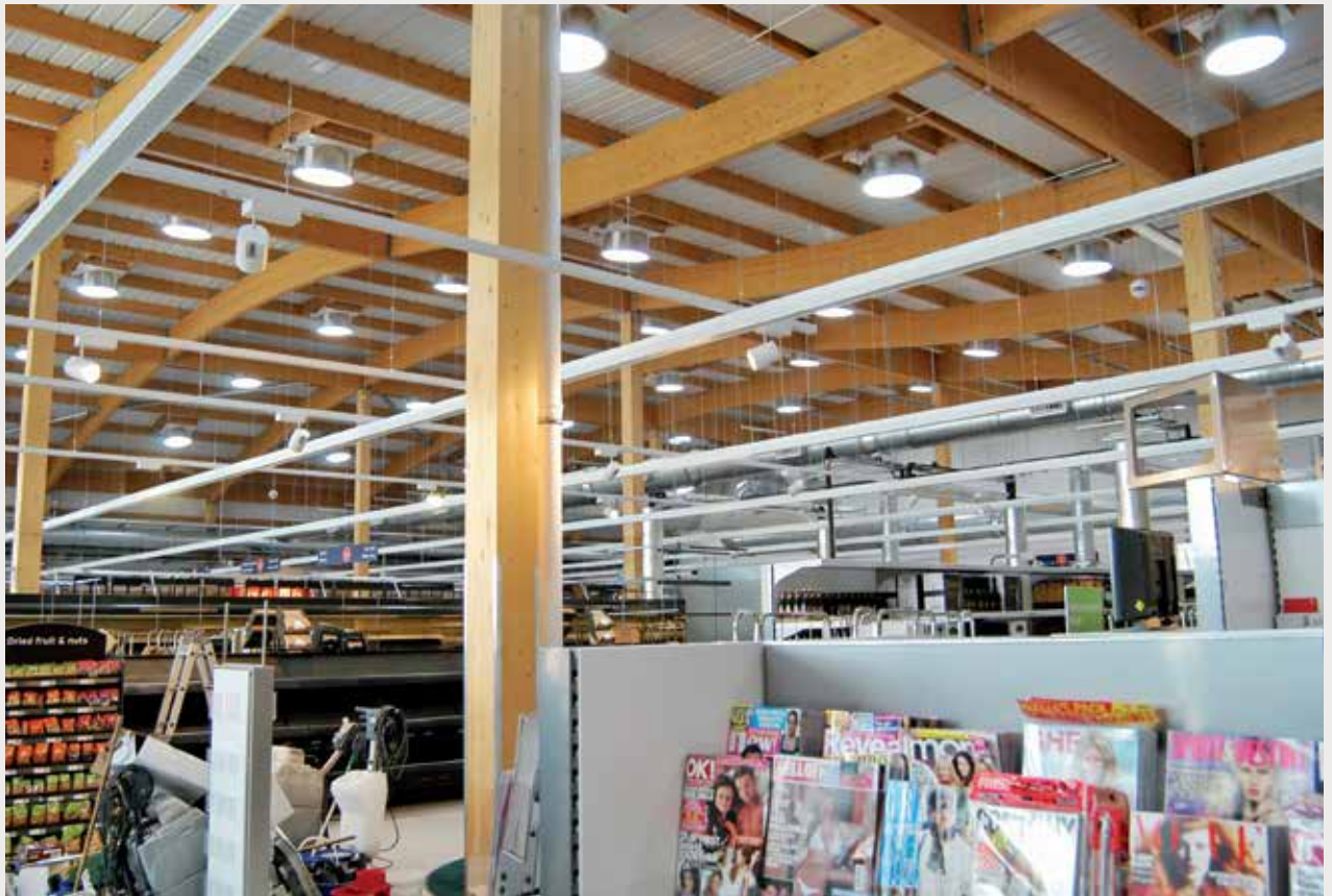
Figure 29: Light pipes used in the sales area, combined with daylight-based dimmable electric lighting, help reduce the energy use significantly (© Monodraught)
