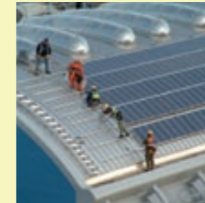
Fitting photovoltaic panels to Newcastle University's Devonshire Building (courtesy of Newcastle University)
