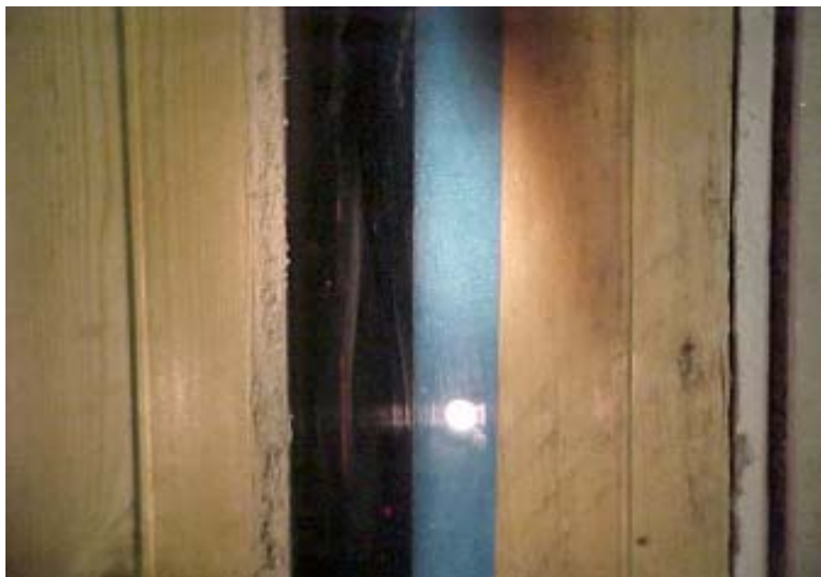
Photograph C3. Showing distortion of the window frame.
