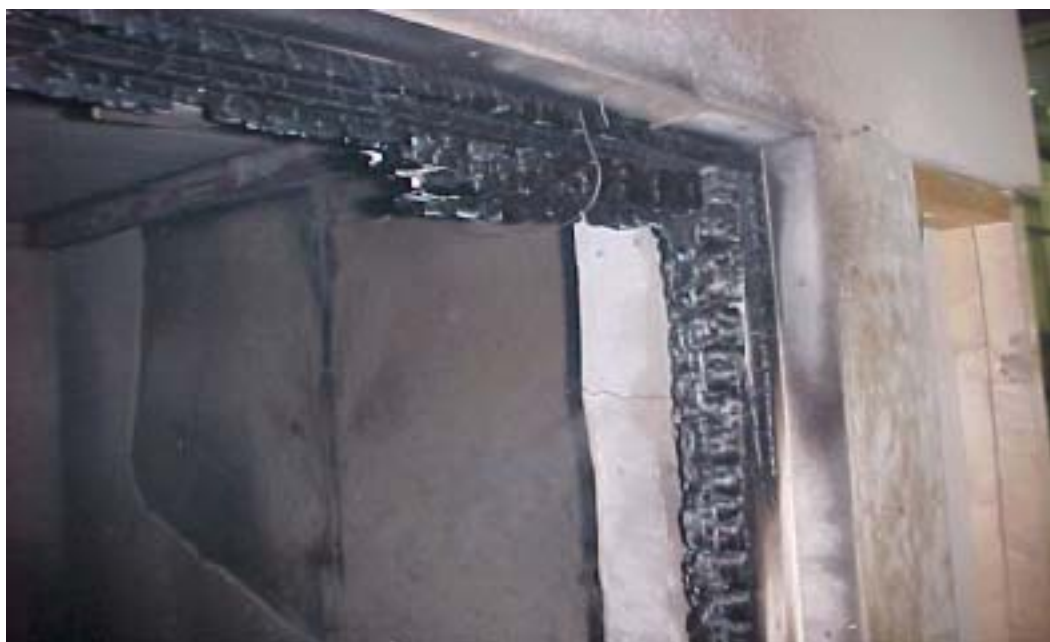
Photograph C10. Showing post test damage.
