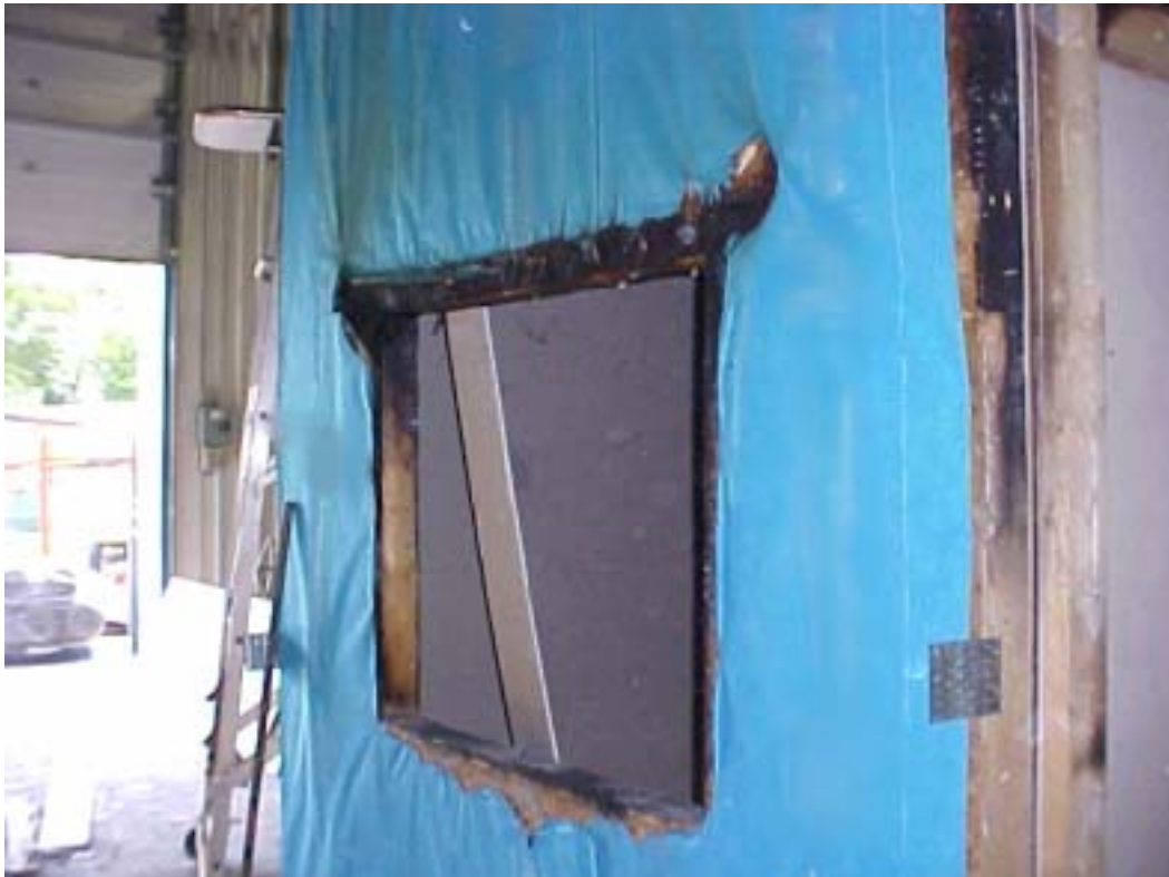
Photograph C13. Showing post test damage.
