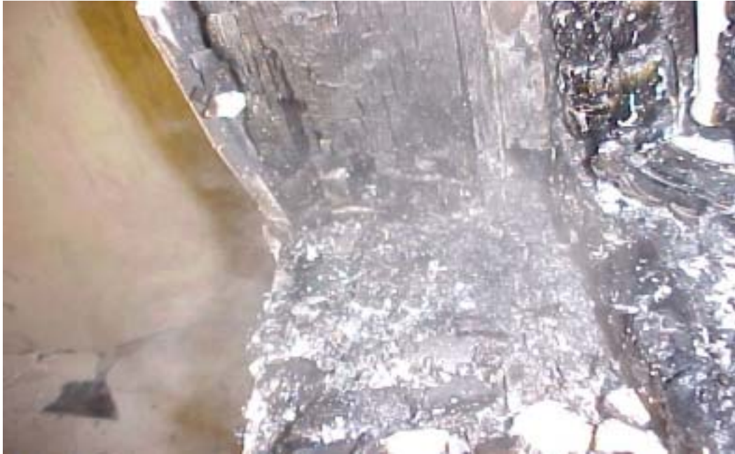
Photograph C12. Showing post test damage.
