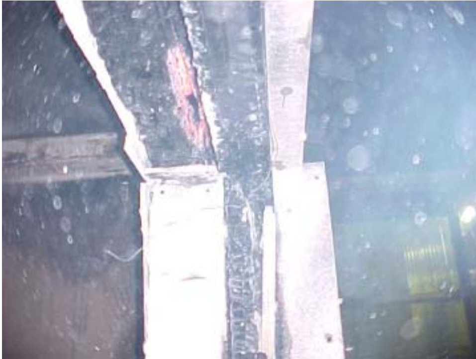
Photograph C8. Showing post test damage.
