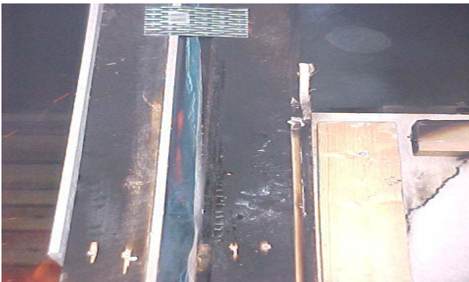
Photograph C7. Showing flaming in the cavity above the window
