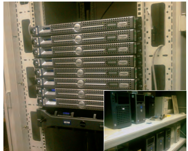
Figure 1: Example of an energy-efficient blade server array. One of these single-blade servers has replaced a bank of traditional servers (see inset, bottom right of photo)
