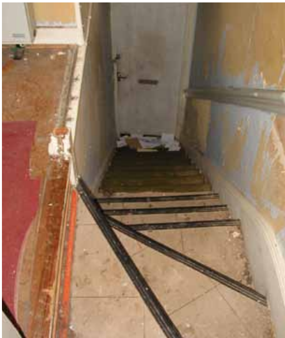
Figure 2: This staircase presents a Category 1 safety hazard
