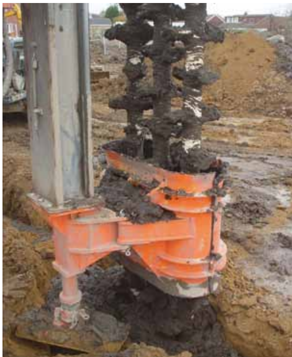
Figure 2: Deep soil mixing using a triple auger system to improve weak soils. Courtesy of Eco Foundations
